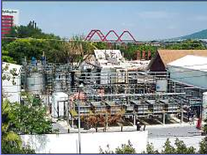
DP, Monterrey, Penoles + Mintek
